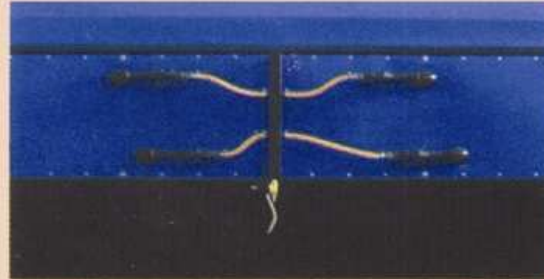
Gas Control Panel
